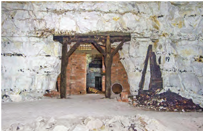
A brick wall separates the mine from the Council repository, while one of the steel sheeted secure enclosures is seen through the door. In front of the wall a chalk roof overhang is propped with more conventional timber mine props. Also visible are exposed steel reinforcement above the concrete door lintel and a large diameter pipe hole, both unusual features whose function is unknown
